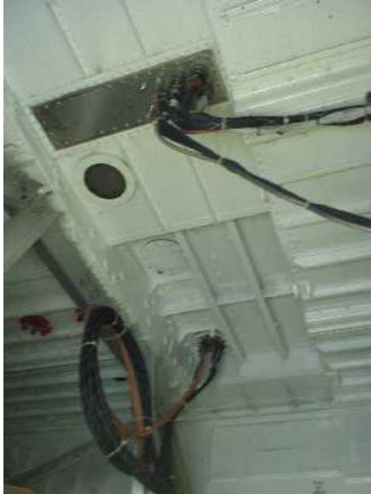
Figure 6: View from just inside open access shown in Figure 4, looking up (toward the floor of the cabin) and slightly forward. The bundle of cables towards the top of the picture is for PSR, and the bundle of cables towards the bottom is for ESTAR.
