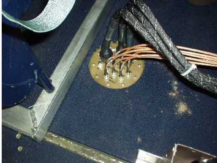
Figure 7: ESTAR cables emerging into cabin area. The diameter of the circular bulkhead is 7\text{-}\frac{3}{8} ".
