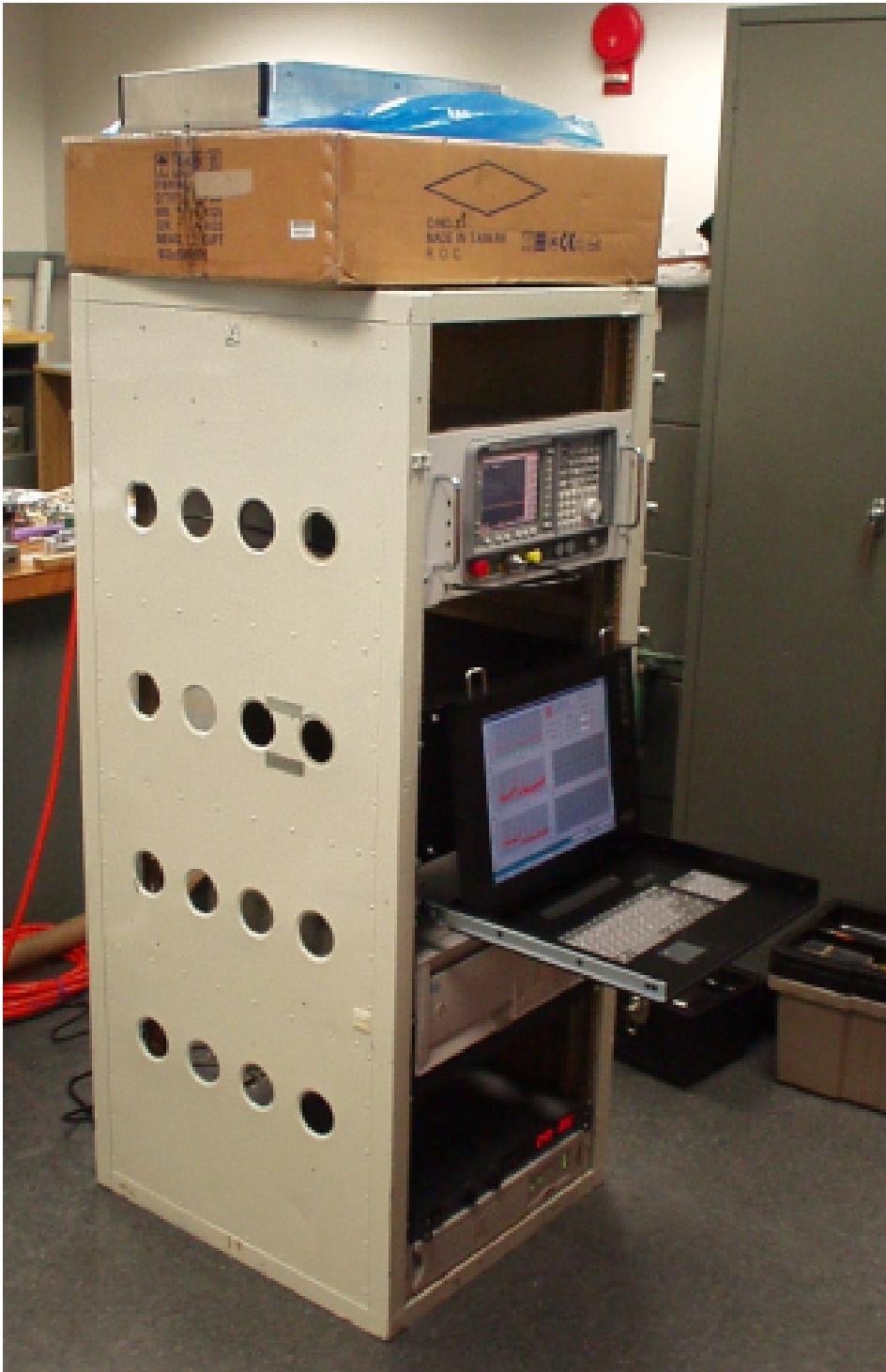
Figure 2: The LISA equipment rack, as it appears when the system is running. (Note that the cardboard box, blue plastic bag, and metal enclosure (actually, the AFEU) are not part of the equipment rack and just happened to be stacked there when this picture was taken.)
