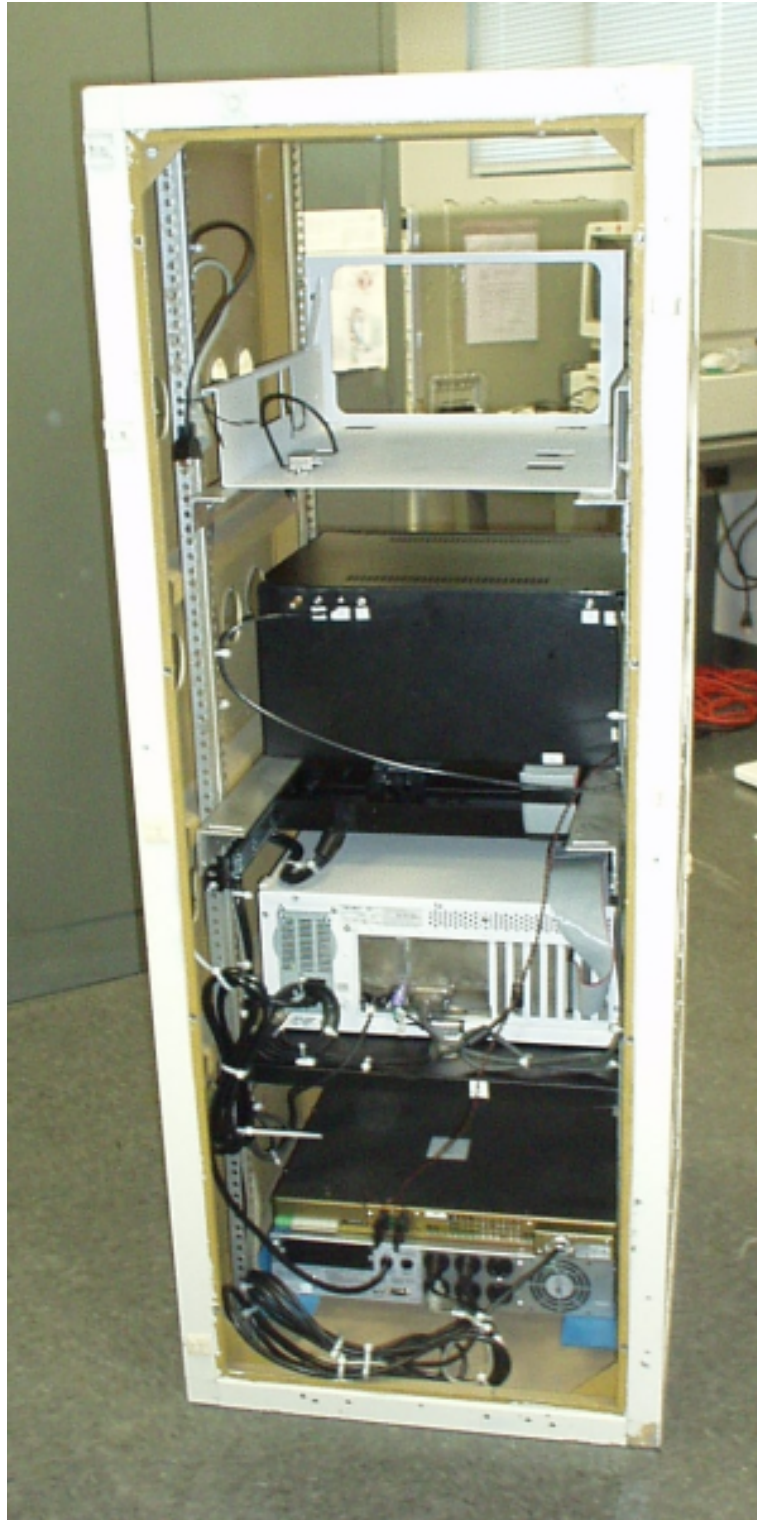
Figure 4: The rear of the LISA equipment rack, as it appears when the system is stowed.
